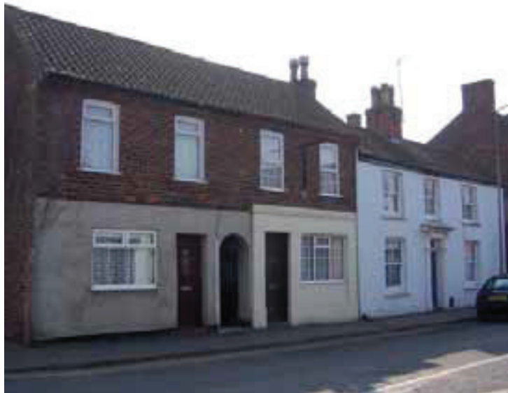
Impact of replacement plastic windows and loss of original slate/pantile roofs
